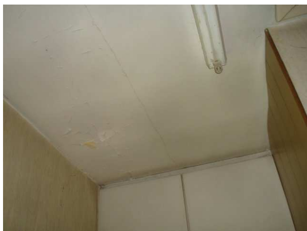
barst in plafond
